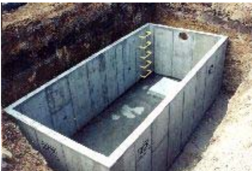
The picture above is an underground tank, before the concrete lid and access grates are constructed.
